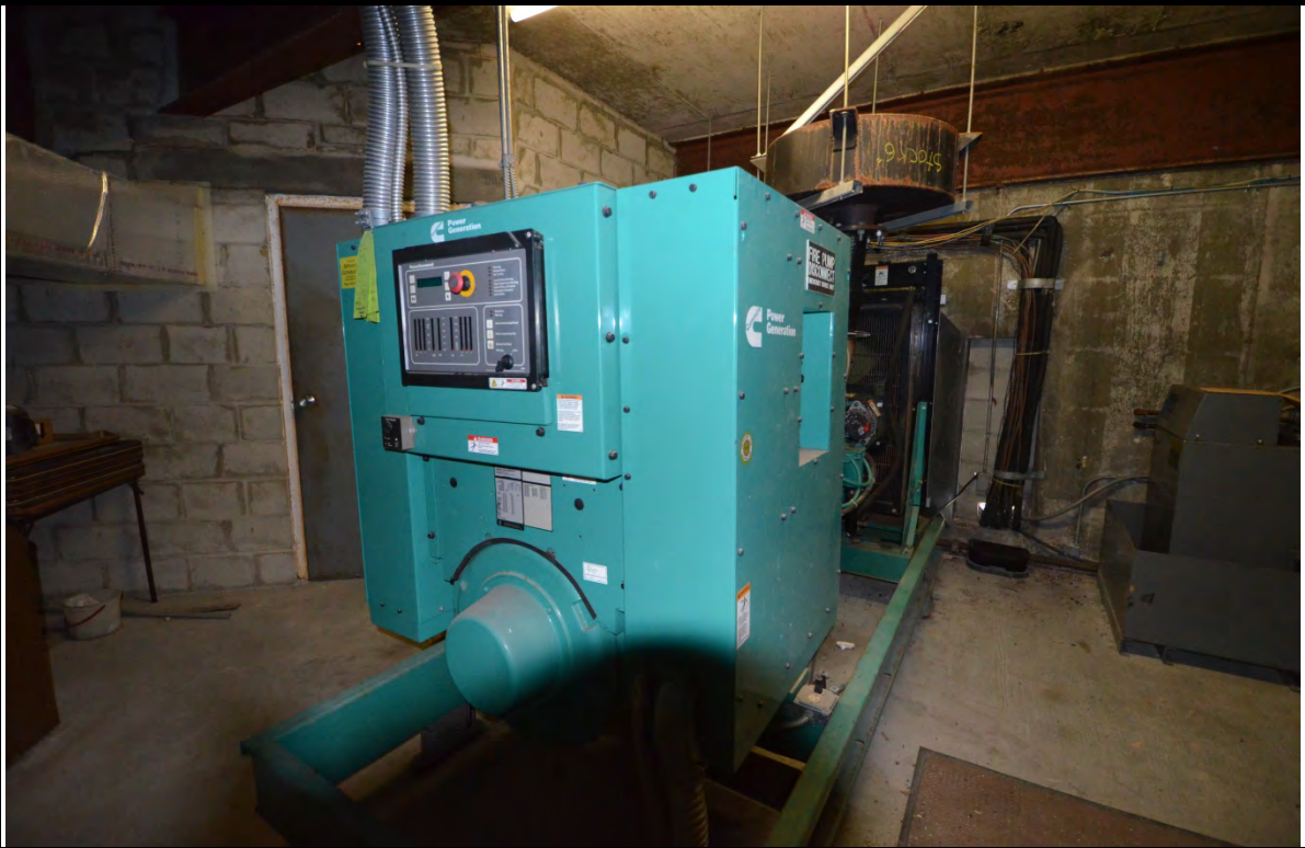
VIEW OF TYPICAL BUILDING MECHANICAL EQUIPMENT
