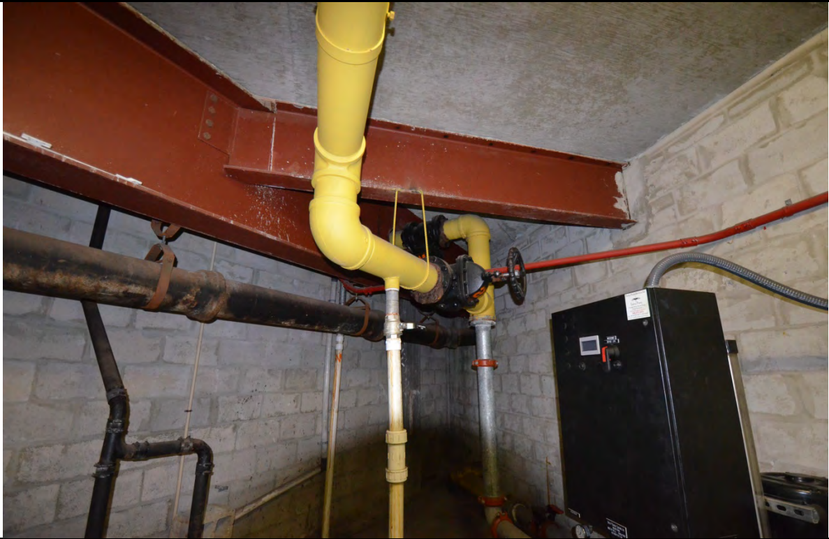
VIEW OF TYPICAL BUILDING MECHANICAL EQUIPMENT
