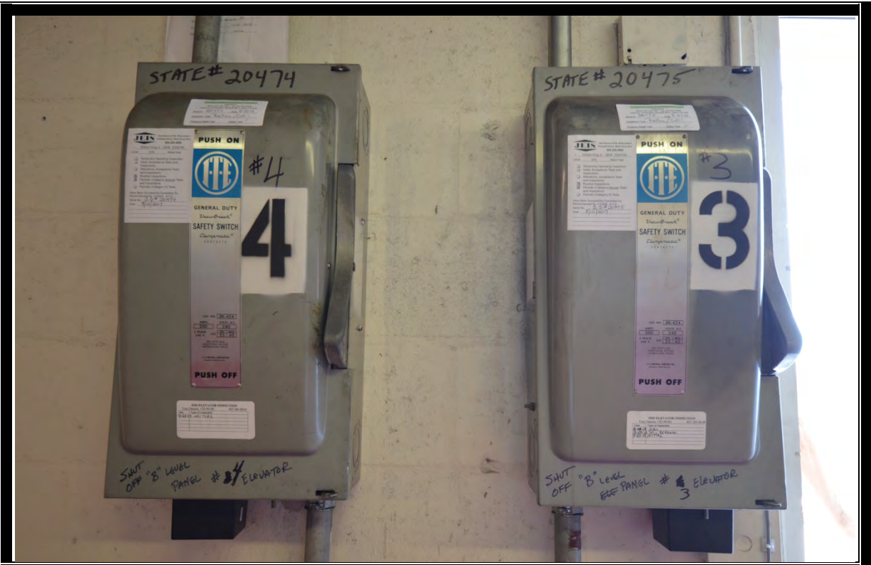
VIEW OF TYPICAL BUILDING MECHANICAL EQUIPMENT
