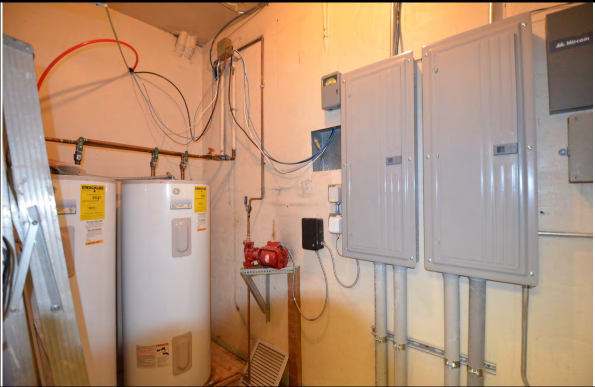
VIEW OF TYPICAL BUILDING MECHANICAL EQUIPMENT
