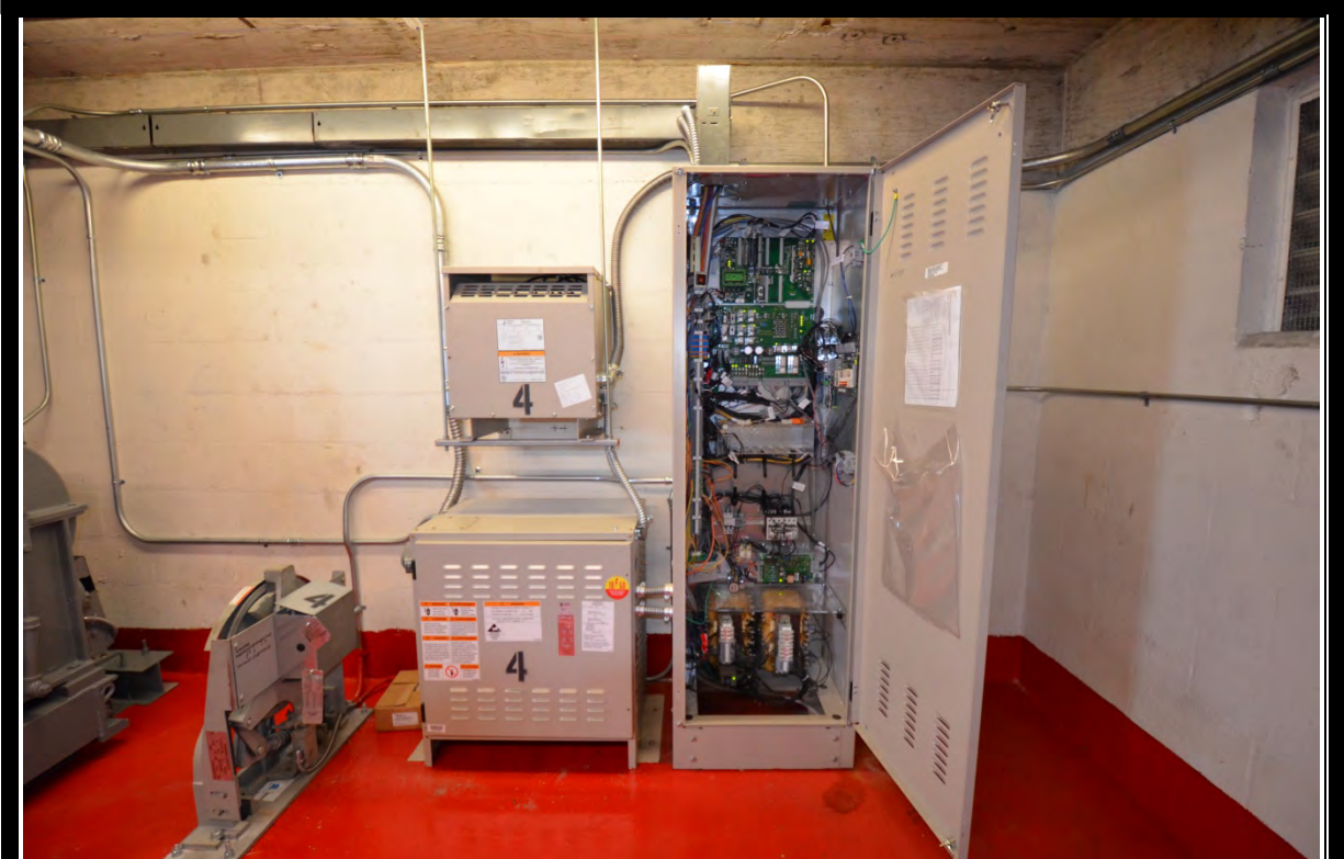
VIEW OF TYPICAL BUILDING MECHANICAL EQUIPMENT
