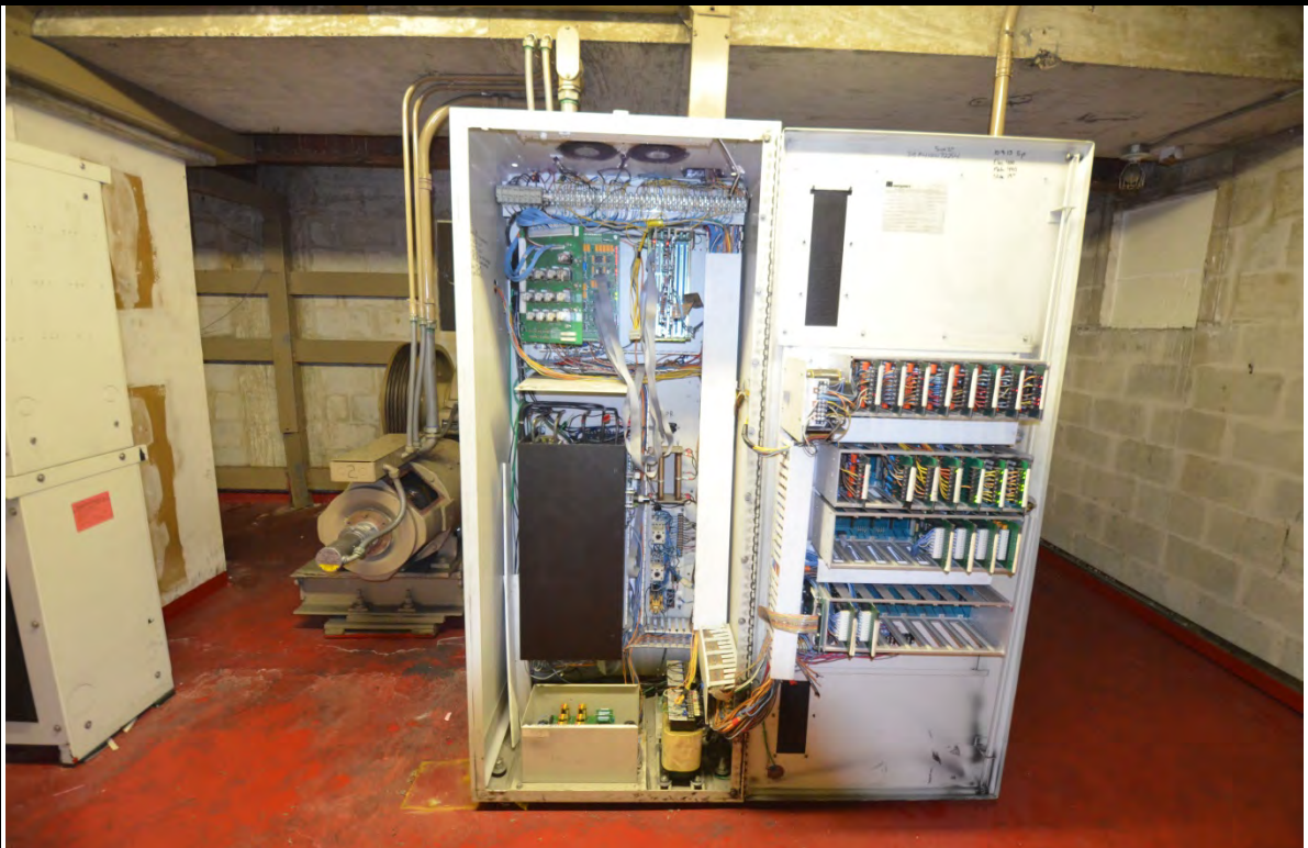
VIEW OF TYPICAL BUILDING MECHANICAL EQUIPMENT
