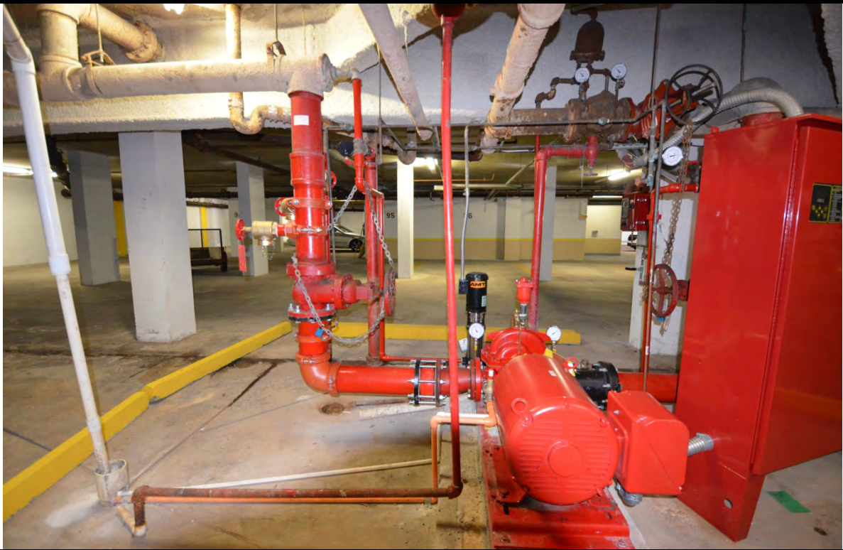
VIEW OF TYPICAL BUILDING MECHANICAL EQUIPMENT
