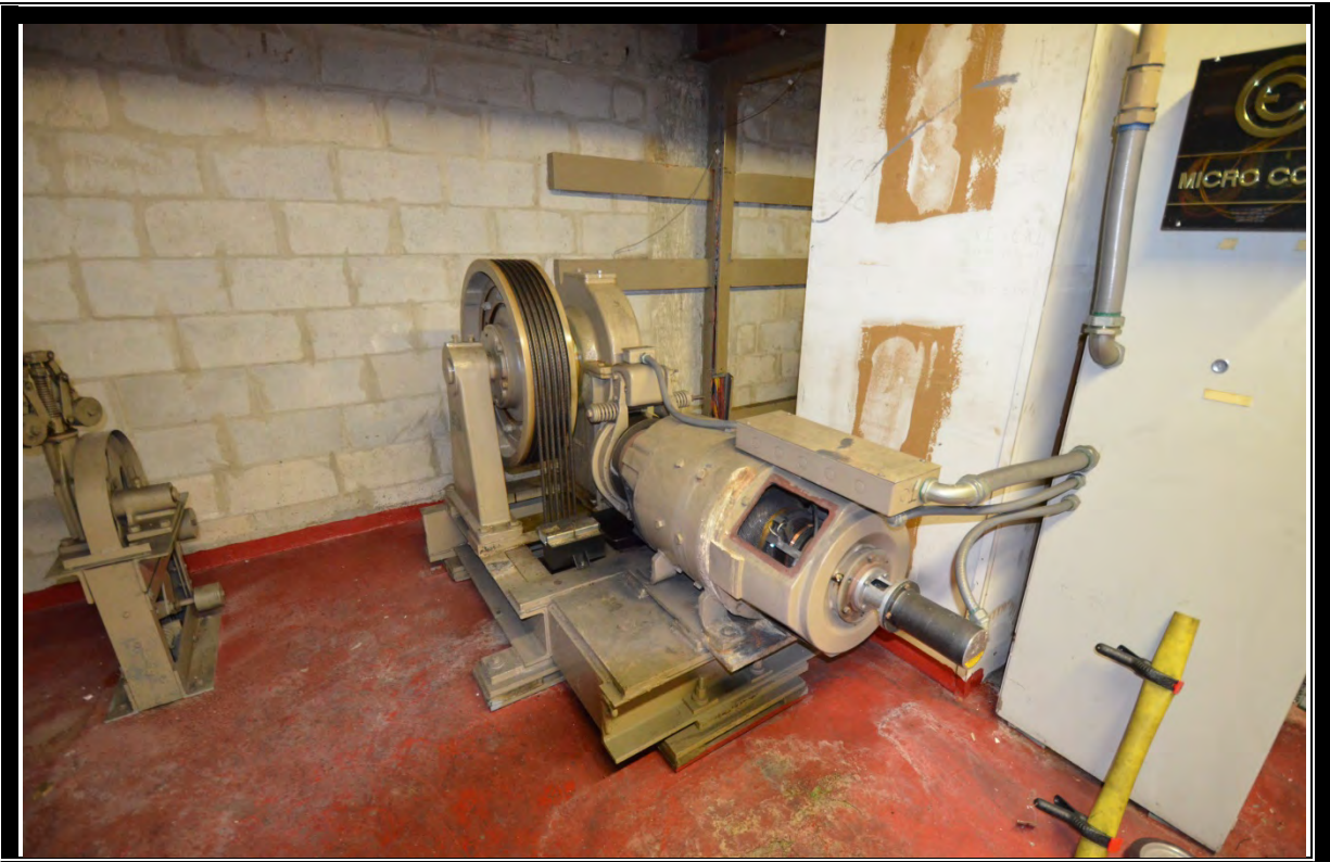
VIEW OF TYPICAL BUILDING MECHANICAL EQUIPMENT
