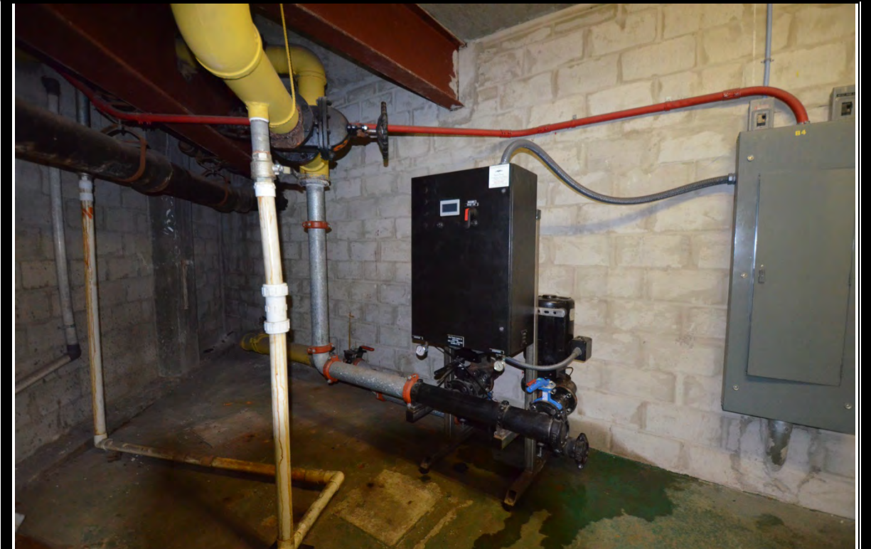
VIEW OF TYPICAL BUILDING MECHANICAL EQUIPMENT
