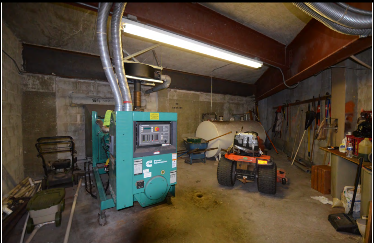
VIEW OF TYPICAL BUILDING MECHANICAL EQUIPMENT
