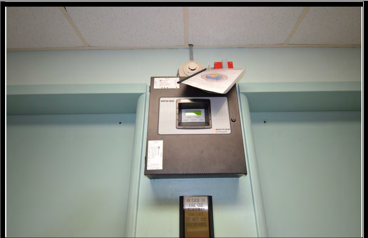
VIEW OF TYPICAL BUILDING MECHANICAL EQUIPMENT
