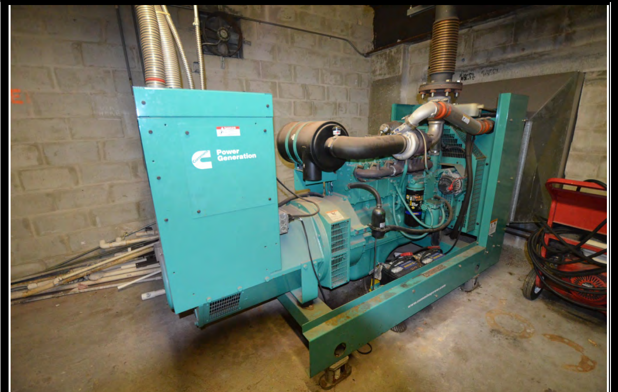
VIEW OF TYPICAL BUILDING MECHANICAL EQUIPMENT
