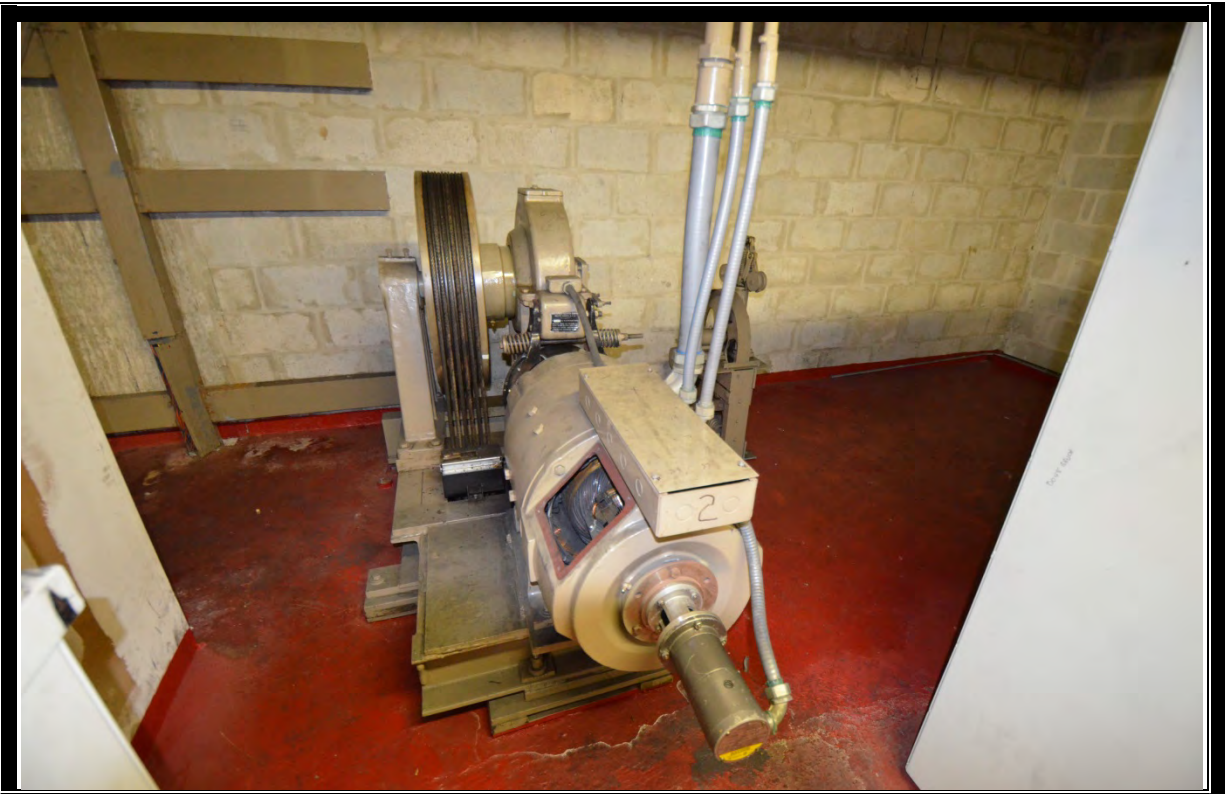
VIEW OF TYPICAL BUILDING MECHANICAL EQUIPMENT
