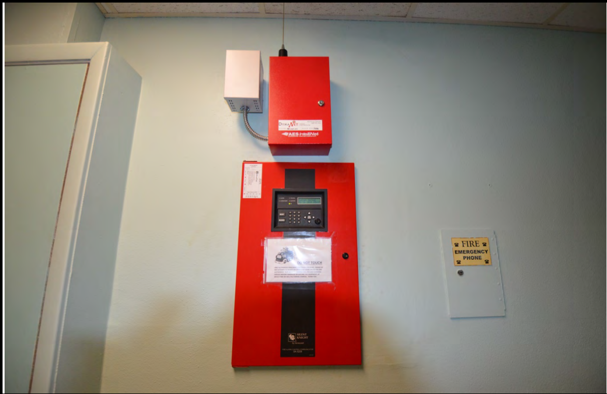
VIEW OF TYPICAL BUILDING MECHANICAL EQUIPMENT
