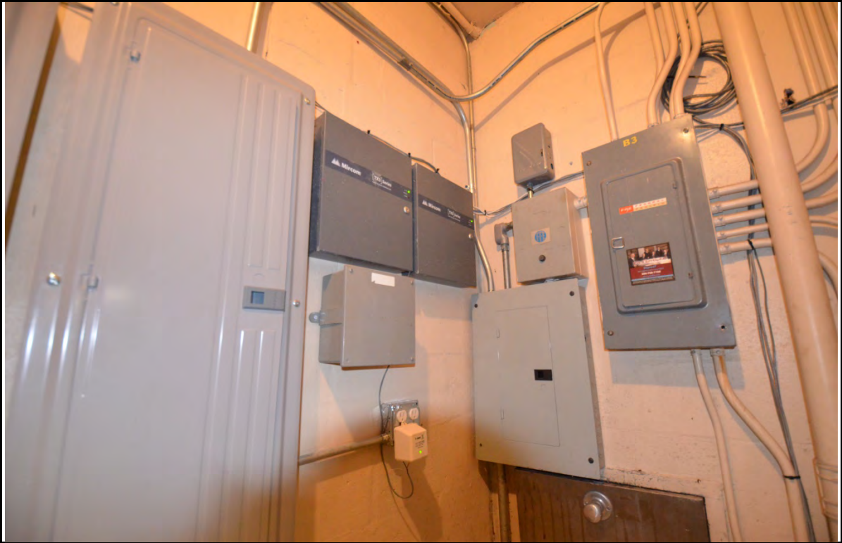
VIEW OF TYPICAL BUILDING MECHANICAL EQUIPMENT
