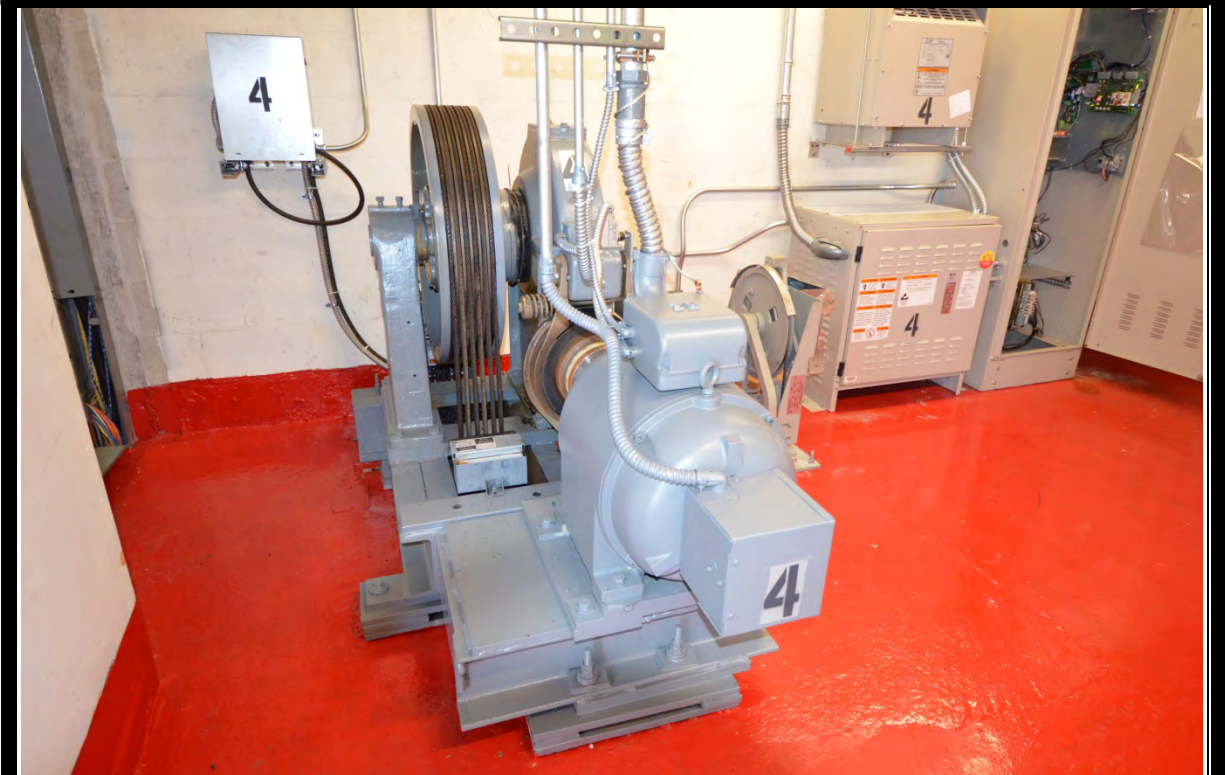
VIEW OF TYPICAL BUILDING MECHANICAL EQUIPMENT
