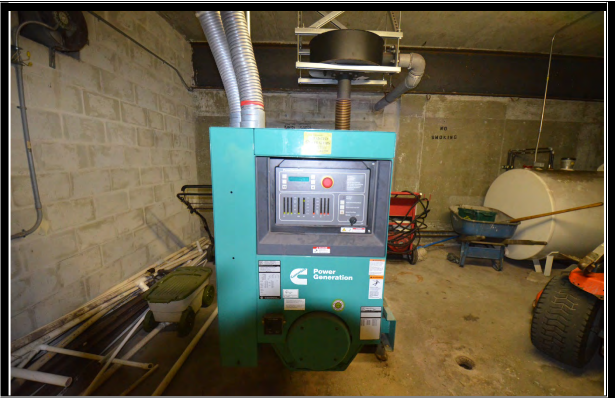
VIEW OF TYPICAL BUILDING MECHANICAL EQUIPMENT
