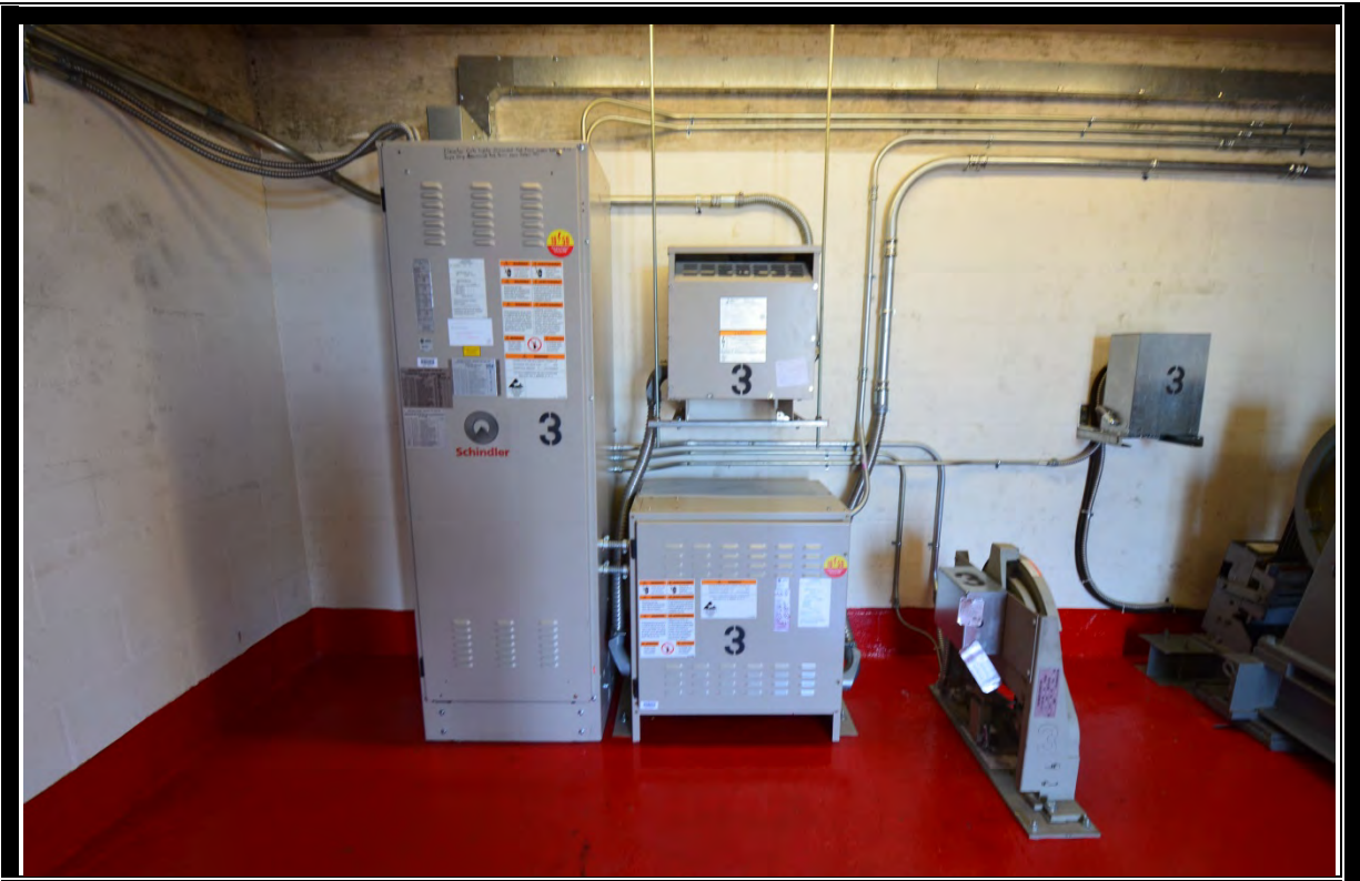
VIEW OF TYPICAL BUILDING MECHANICAL EQUIPMENT
