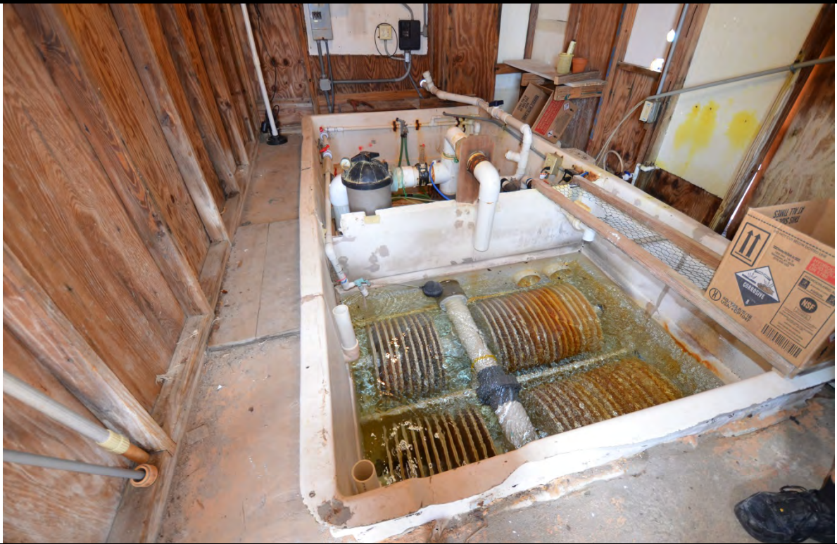
VIEW OF TYPICAL POOL EQUIPMENT
