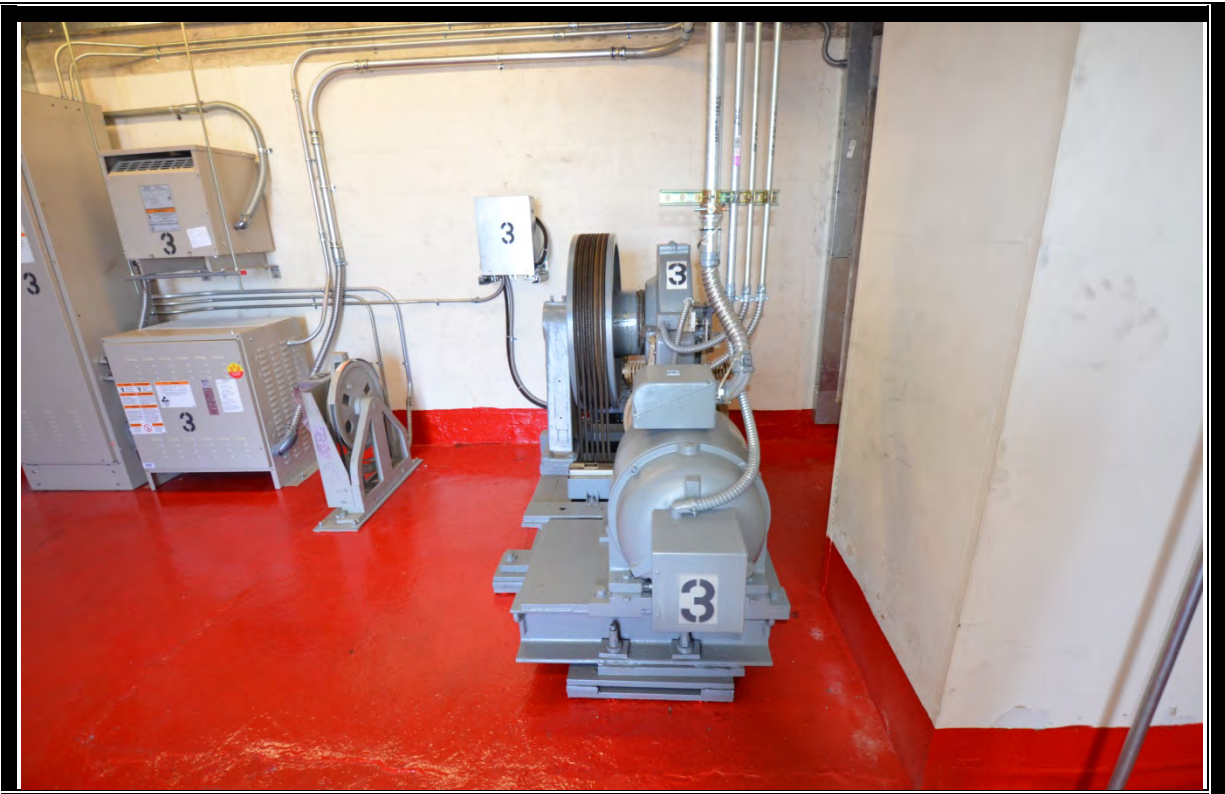
VIEW OF TYPICAL BUILDING MECHANICAL EQUIPMENT
