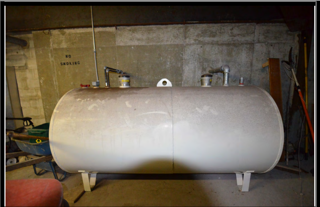
VIEW OF TYPICAL BUILDING MECHANICAL EQUIPMENT
