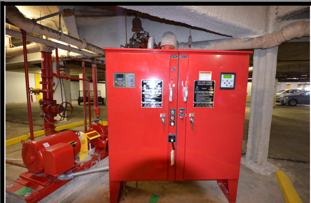
VIEW OF TYPICAL BUILDING MECHANICAL EQUIPMENT
