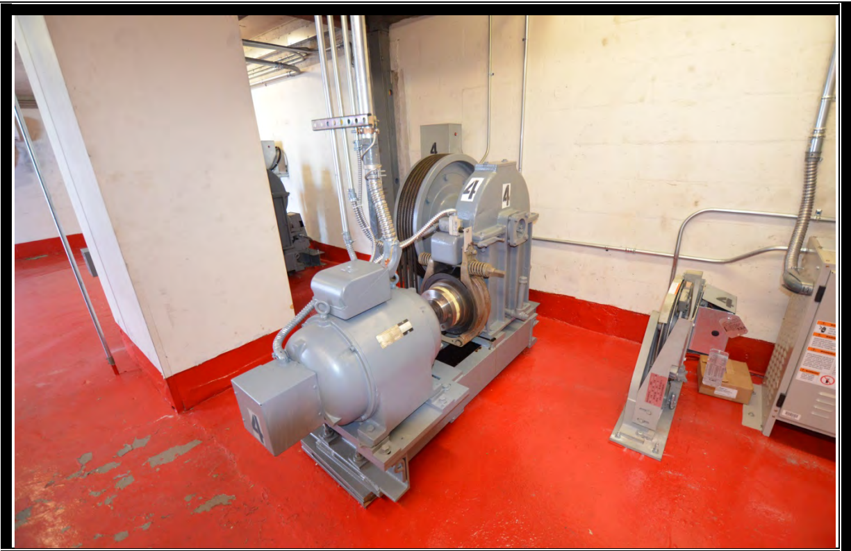
VIEW OF TYPICAL BUILDING MECHANICAL EQUIPMENT
