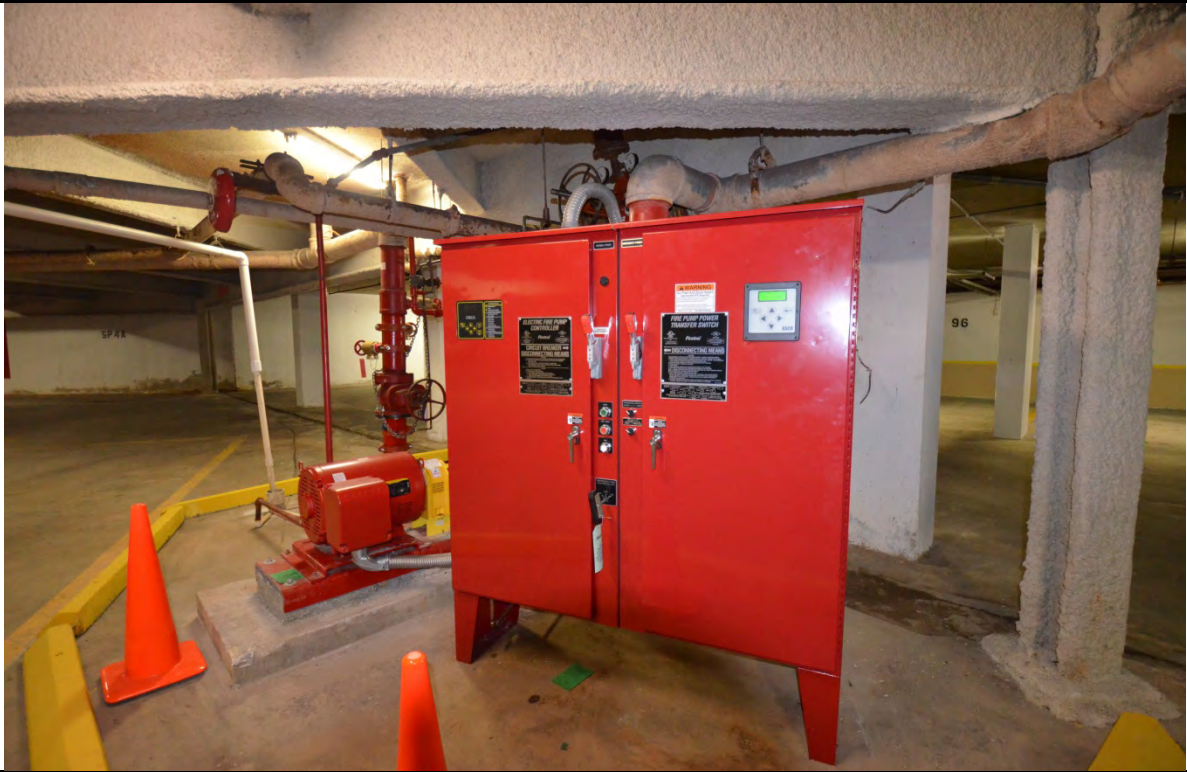
VIEW OF TYPICAL BUILDING MECHANICAL EQUIPMENT
