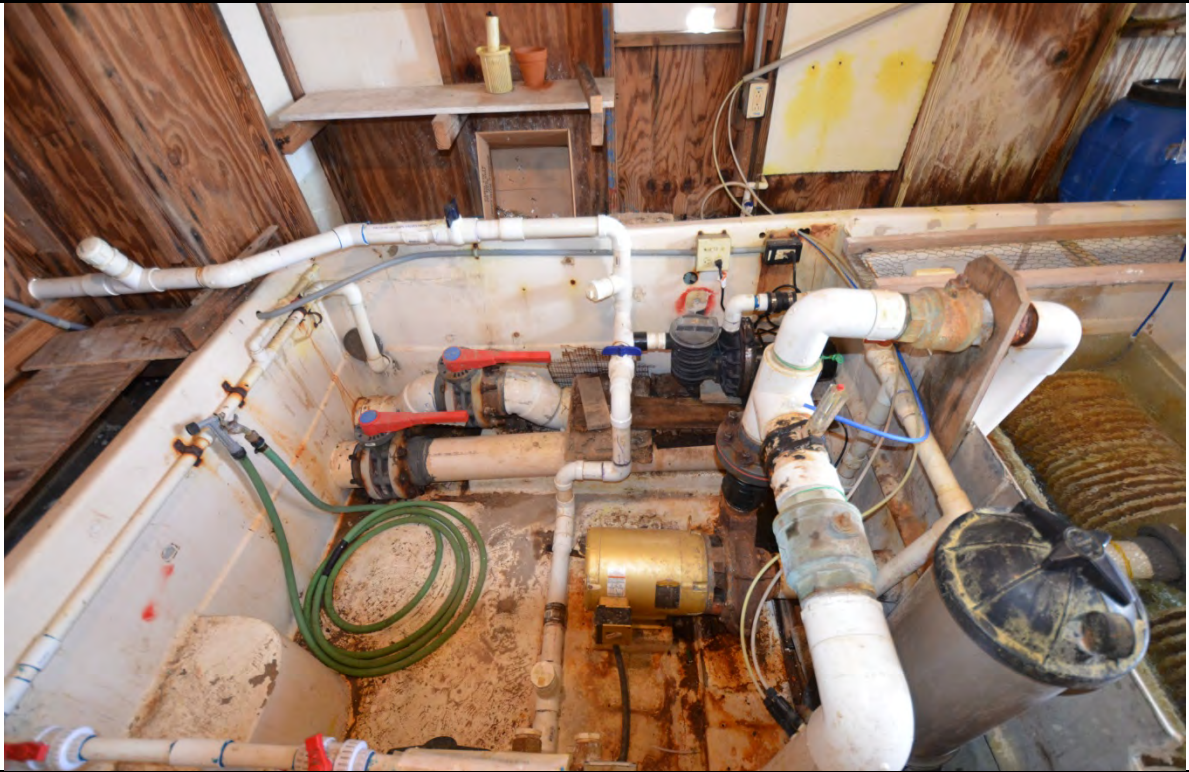
VIEW OF TYPICAL POOL EQUIPMENT
