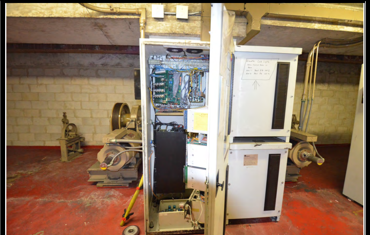
VIEW OF TYPICAL BUILDING MECHANICAL EQUIPMENT
