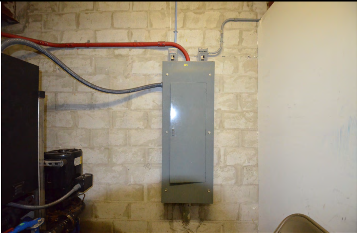
VIEW OF TYPICAL BUILDING MECHANICAL EQUIPMENT
